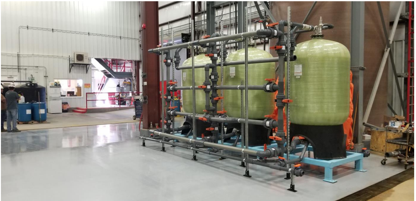
Figure 2: Constructed Ion Exchange Test Columns for MU1A field demonstration
