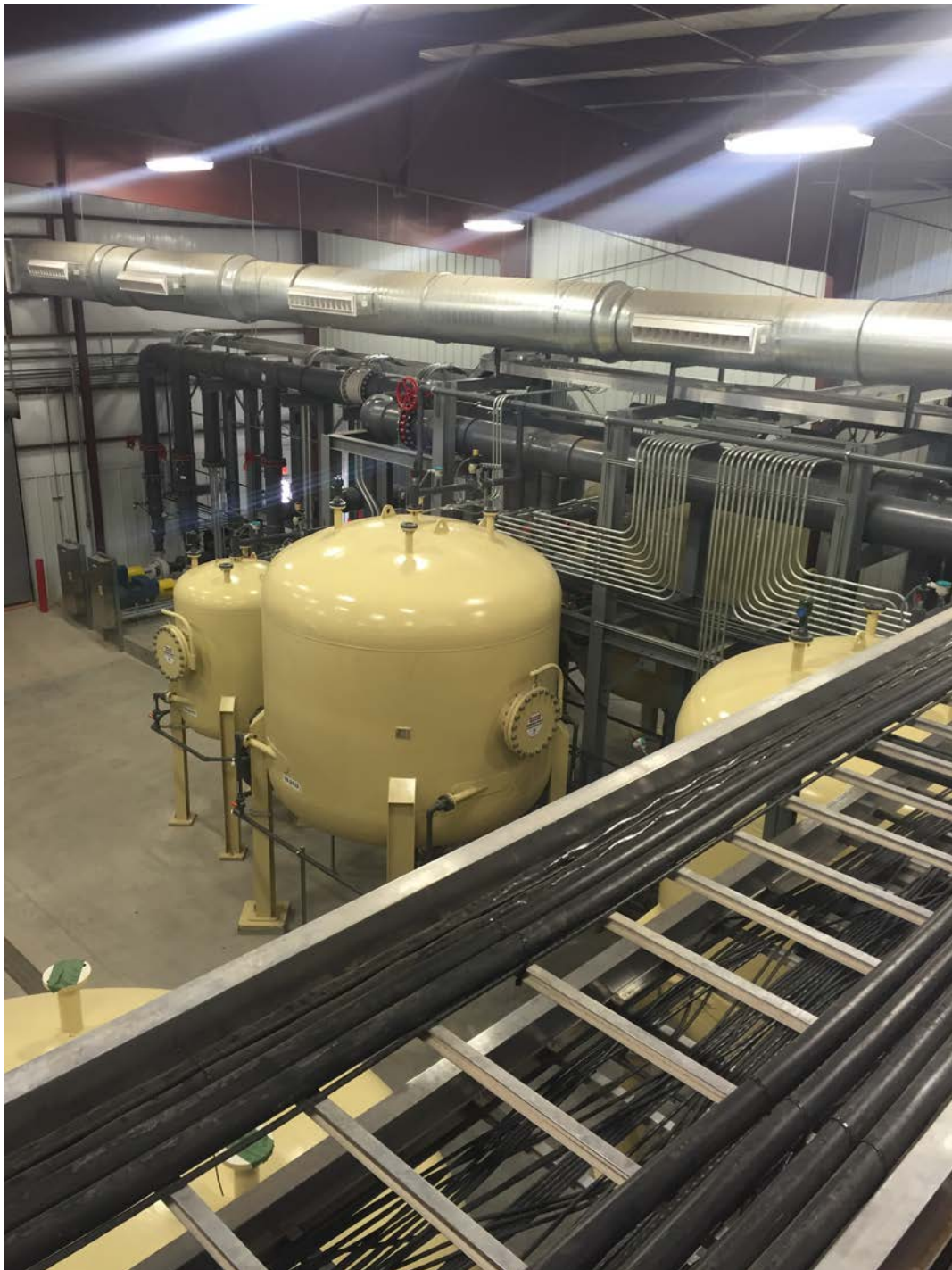
Figure 5: Inside operating Central Processing Plant – December 2015
