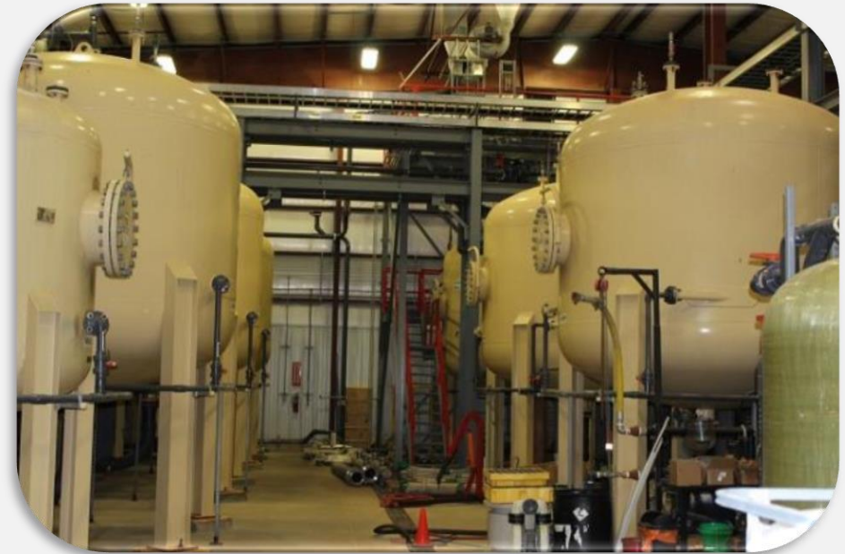
Lance Satellite Plant Ion Exchange System
