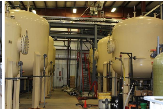
Process plant to be activated for production activities for mid-year 2023
